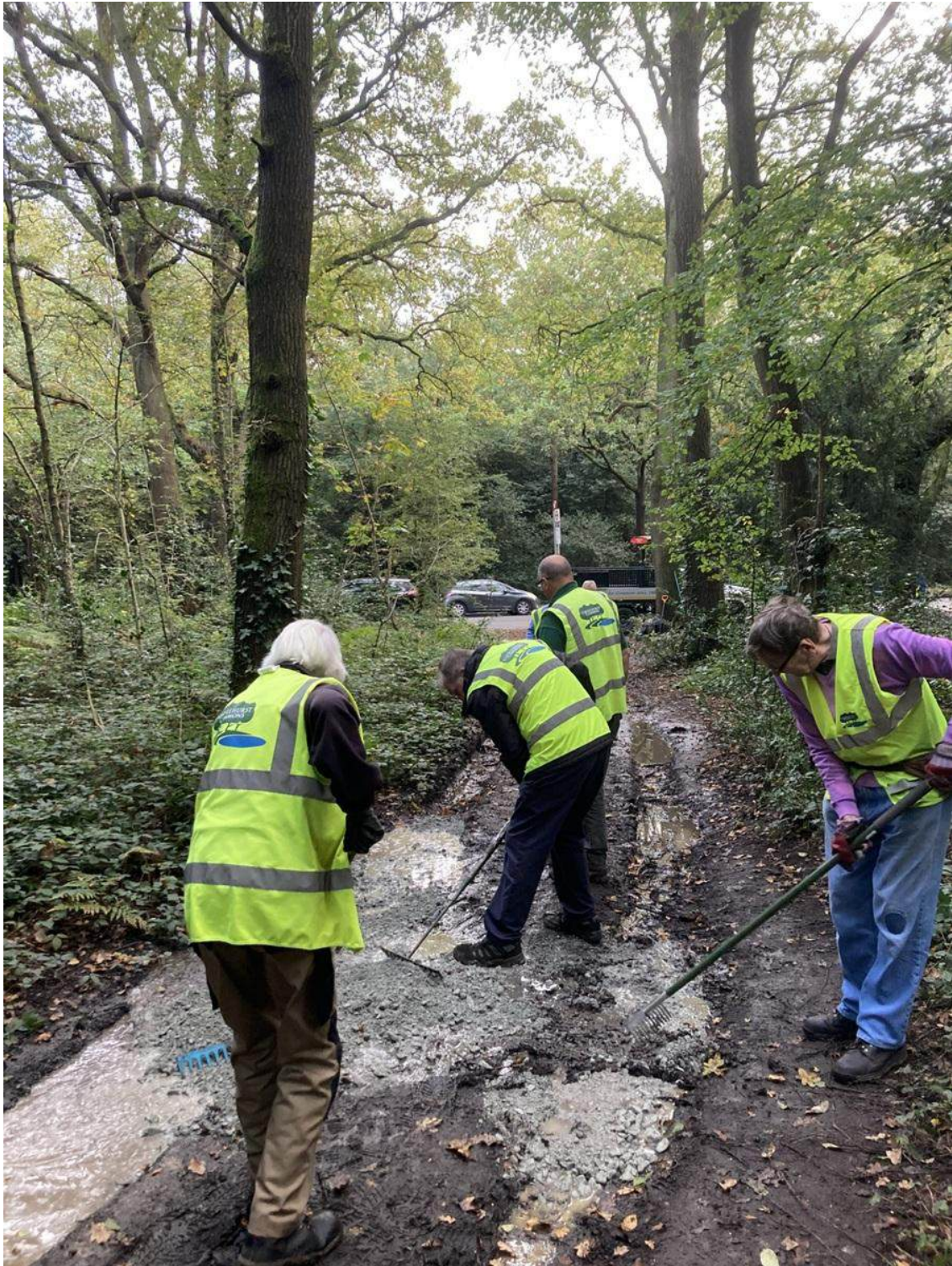
Path maintenance is another task for the volunteers before winter sets in. Here they are repairing the footpath from the bus stop at the War Memorial.
